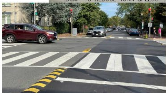
636 INSTALL LOW PROFILE SPEED BUMP TO REDUCE TURN SPEEDS
